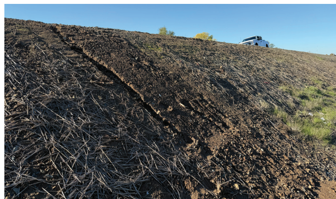
Rainfall erosion on levee.
