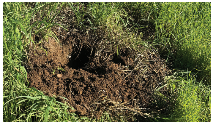
Rodent burrow damage on levee.
